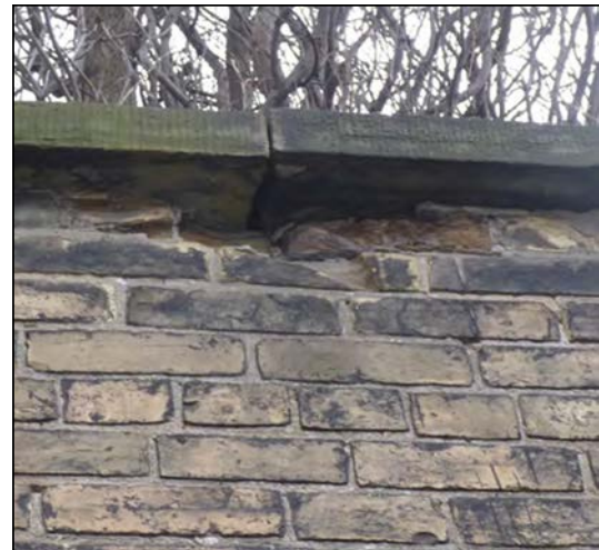
Typical deterioration of brickwork under open joints in cap stone
