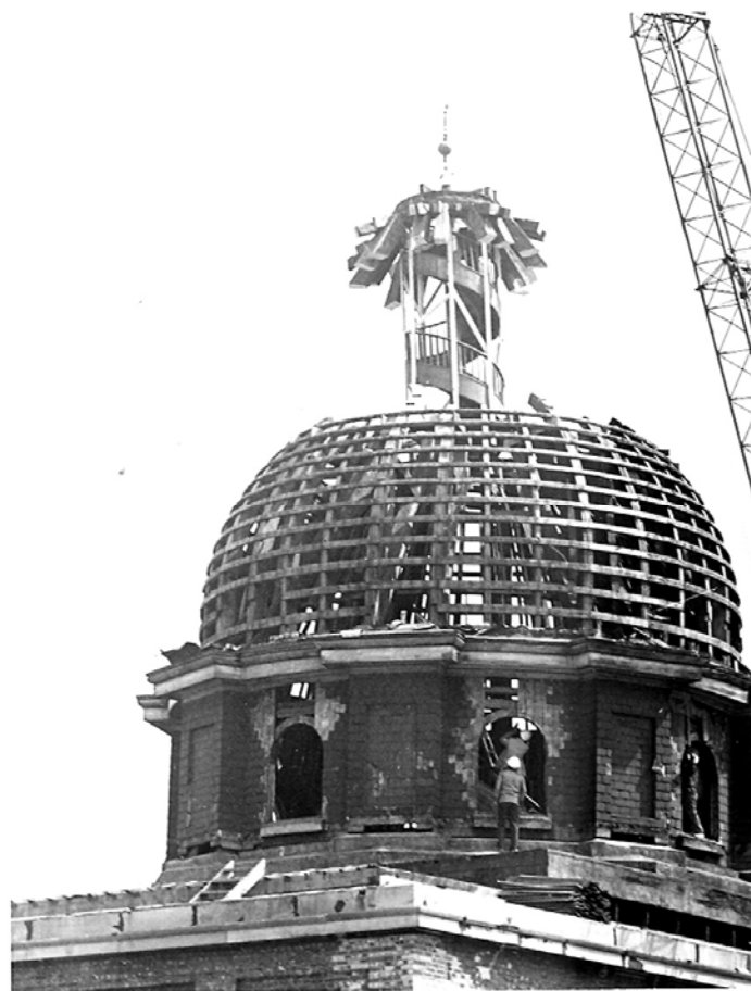
During demolition in 1976 of the original Queen Street asylum structure, built 1846-50, a crane extracted the “flying staircase” for preservation as an artifact. Photo print: CAMH Archives, Queen Street fonds, 32-21.
